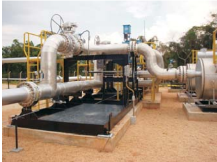
City Gate instalado
